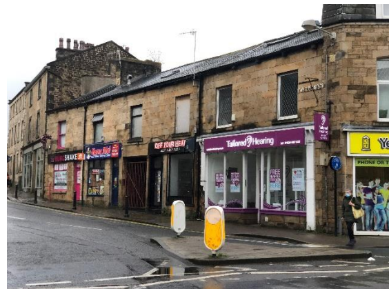
Figure 10: This terrace of purpose-built early C19 shops on St Leonard's Gate could make a highly positive contribution to the area but it suffers from being in poor condition and from unsympathetic alterations.
