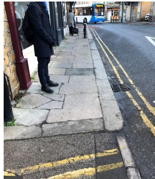
Figure 17: The damaged and infilled footpath on a section of Damside Street
